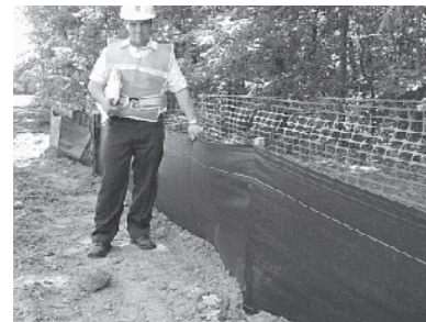
Proper installation and regular inspection and maintenance of erosion and sediment controls are essential for effective resource protection. (Pictured in photo: Mr. Dave Gaspar, Long Island Regional Stormwater Control Specialist).
