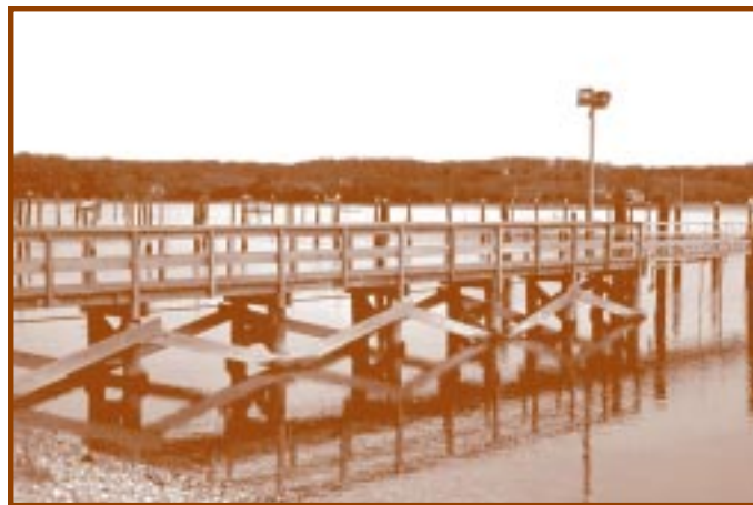
Low tide along this dock on Long Island’s north shore reveals the structure made of treated wood.
